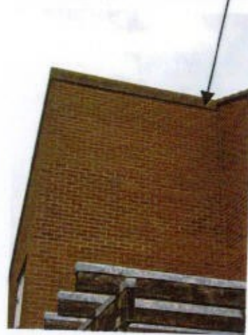
Photograph 9: Fascia board gap
