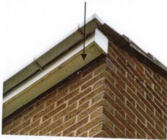
Photograph 8: Gap along soffit boards
